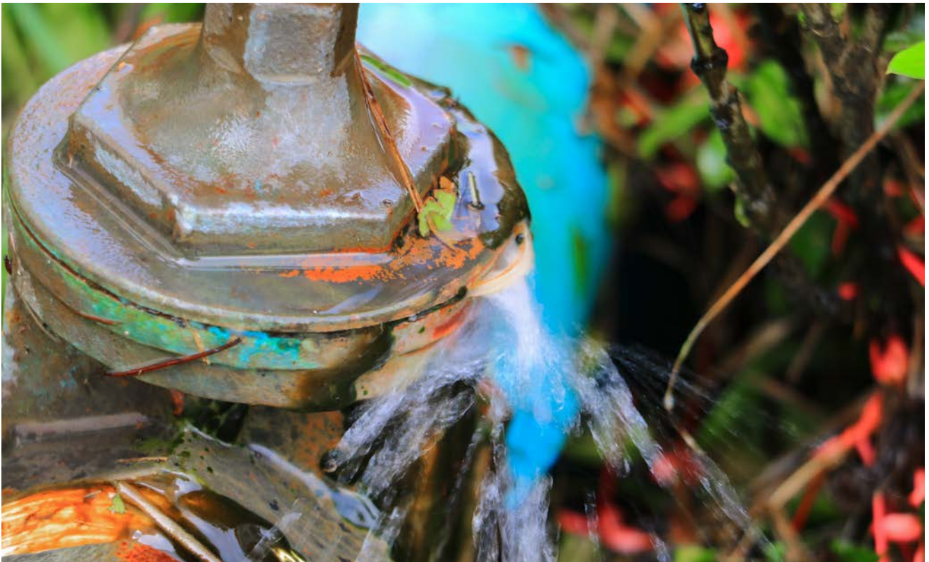
High technical water losses are most likely due to historically poor maintenance and lack of adequate asset replacement leading to old, leaking infrastructure.
