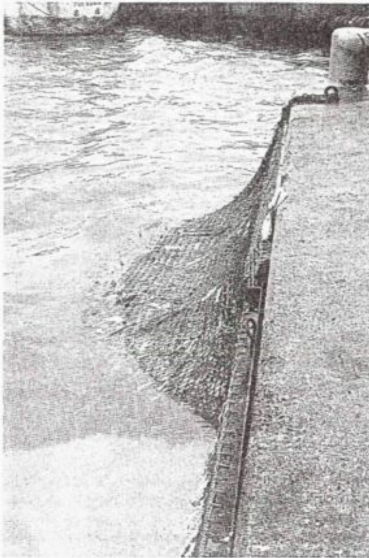
Figure 6-5 : View of the nets over the mouth of the Capel Sloop culverts in the Duncan Docks in Table Bay, Cape Town
