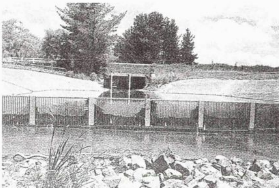
Figure 6-6 : View of a typical Canberra type Gross Pollutant Trap (GPT) looking upstream from below the screen
