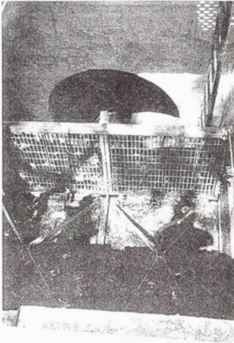
Figure 6-8 : View inside the North Sydney Litter Control Device (LCD)
