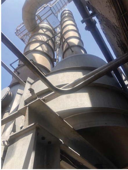
Figure 10-16: Photo Image of Evaporators at West Point Processors
