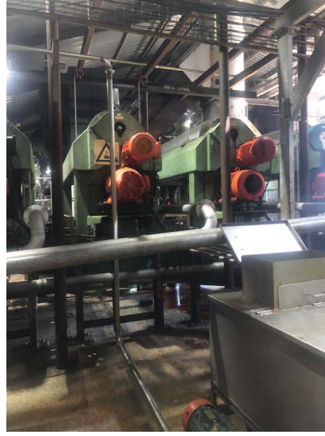
Figure 10-13: Photo Image of Decanting Centrifuges at Lucky Star, St Helena Bay
