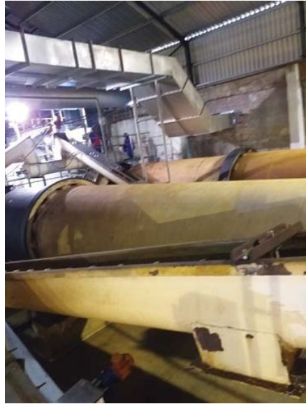
Figure 10-15: Photo Image of Set of Dryers at Gansbaai Marine
