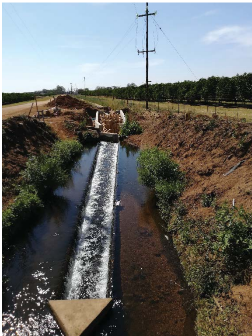
Figure A12: Farm irrigation canal with construction conducted when this photo was taken
