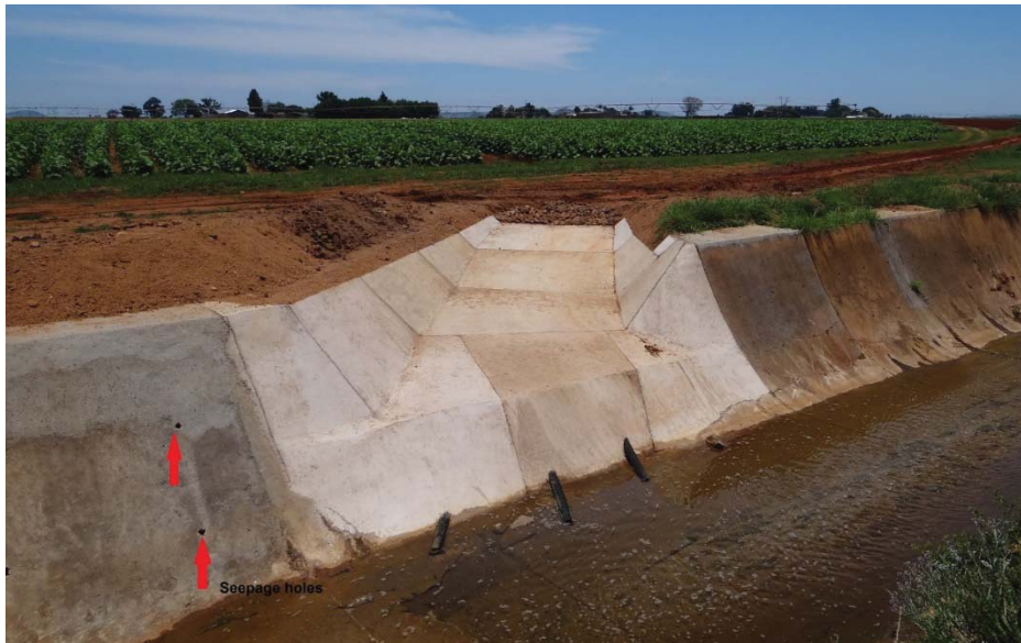
Figure 106: Water entering drainage canal DE1 through seepage holes
