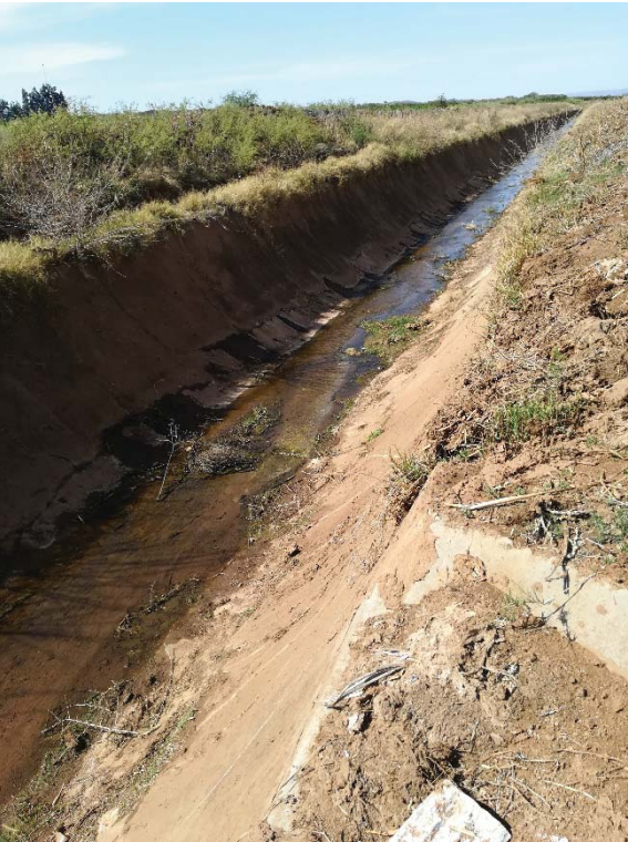
Figure A16: Drainage canal DE10
