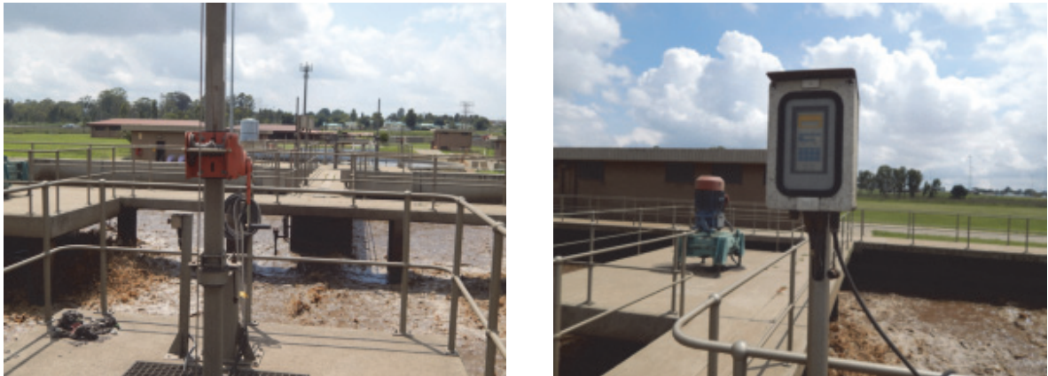
Figure 5-2: JP Marais Surface Aerators
