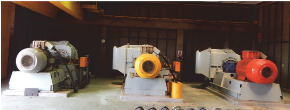
Figure 4-3: Module 1 Single Speed Centrifugal Blowers (Photo Courtesy City of Tshwane)
