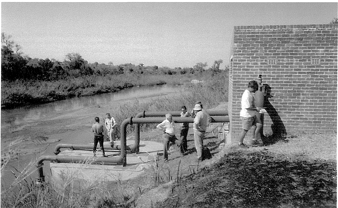
Sand River pump station: Sediment management at intake pumping stations.
