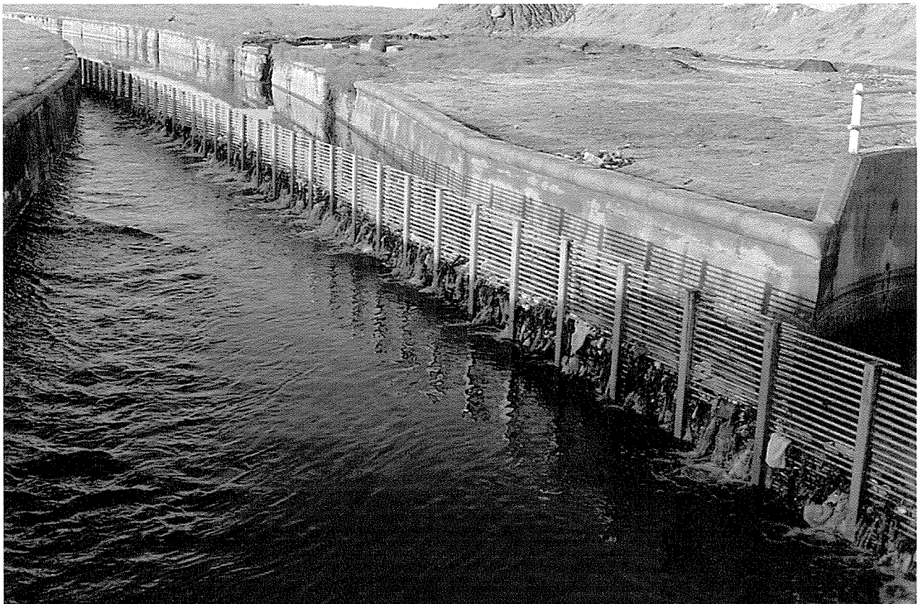
"Enviroscreen" with trash sticking to the screens. Cape Town City Council.
