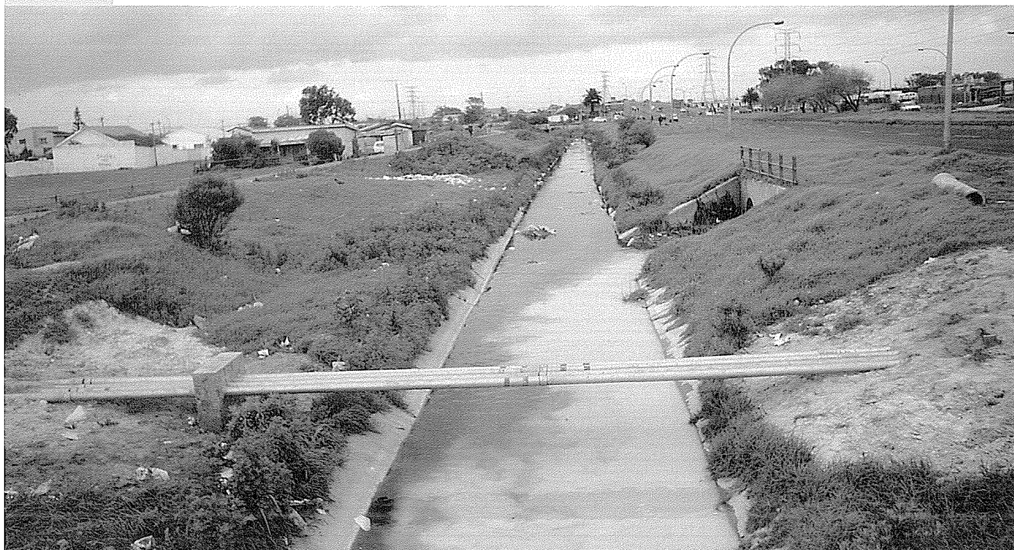
Inflow of polluted stormwater into the Lotus River from Philippi East (construction work/paint). Note polluted stormwater, dumping and littering, and unnecessary and unsightly service conduit for electricity which could have been routed along pedestrian bridge.
