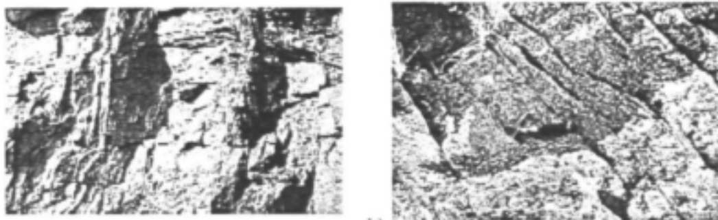
a) Oribi Gorge porphyritic granite (Stop 49), with two near vertical dip-slip, Mode 1 joint sets.
