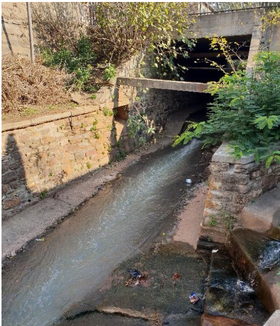
Source of the Jukskei River contaminated by sewage entering groundwater
