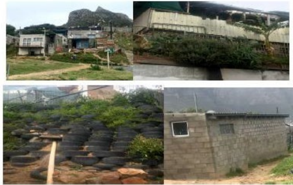
Figure 52: Different structures in Hangberg to deal with flooding and unstable slopes (source: Faith Gara)
