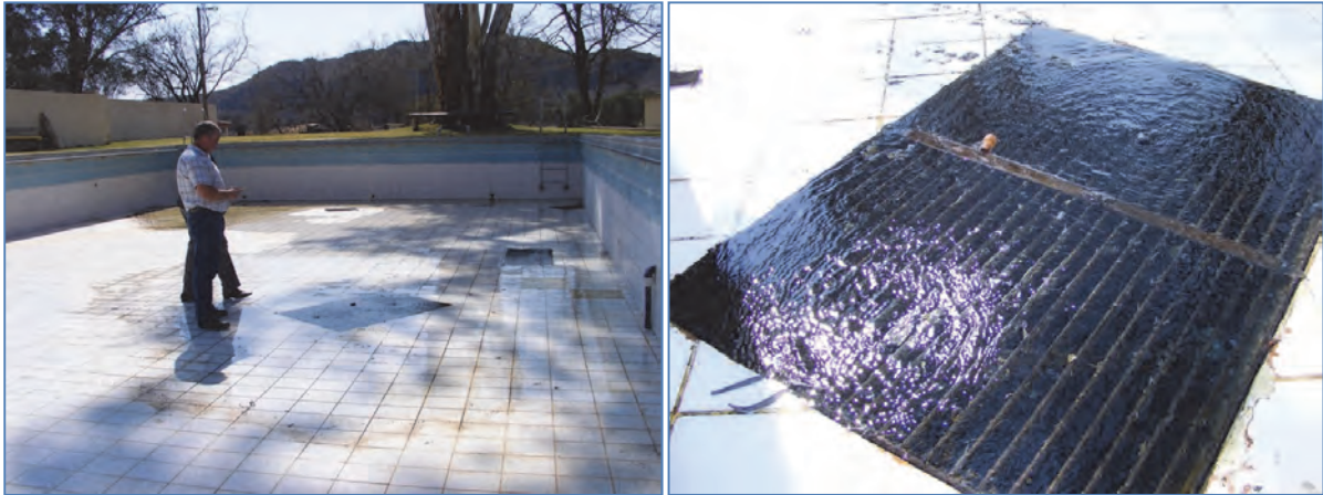
Figure 15: Cradock spa swimming pool in August 2013 (after being drained for cleaning), with metal grids protecting the bubbling springflow from below (photo courtesy S Mullineux, DWA, Cradock).
