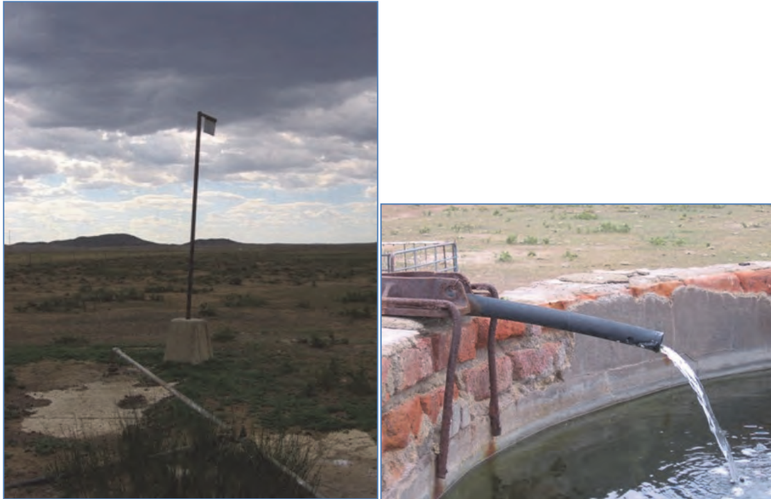
Figure 4: The Trompsburg artesian borehole (located to the left of the beacon), and discharging into a brick reservoir.
