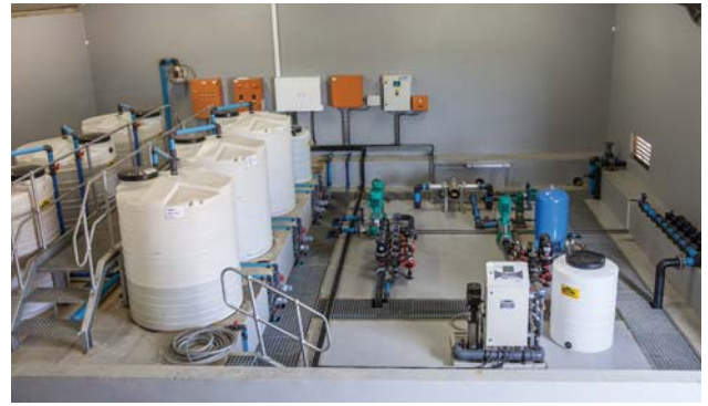
Part of the new system includes that all valves fertilizer is moved to a central pump house.
