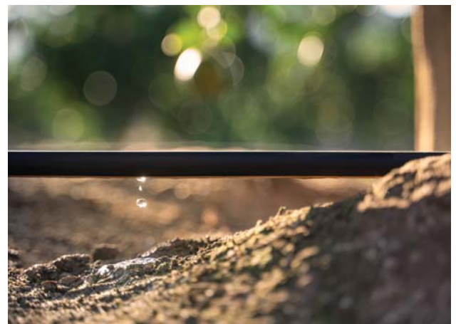
Dripperline for a low flow irrigation system.
