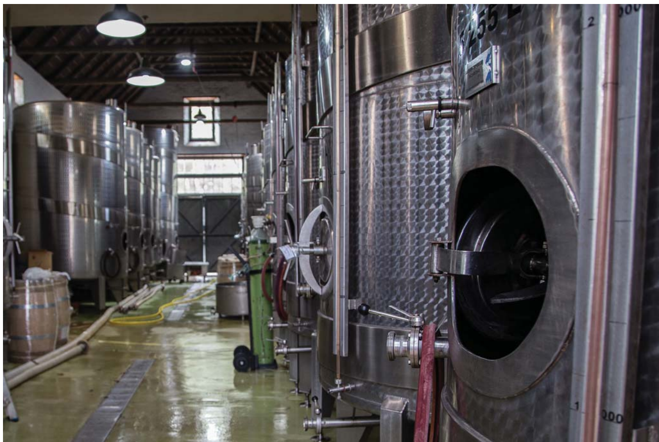
Most of the wastewater generated by wineries is from the cellars, and is generated during the production process.
