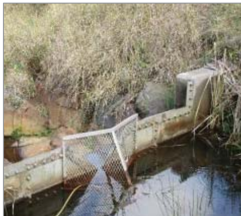
Figure 5.6 Compound V-notch weir located at Two Streams
